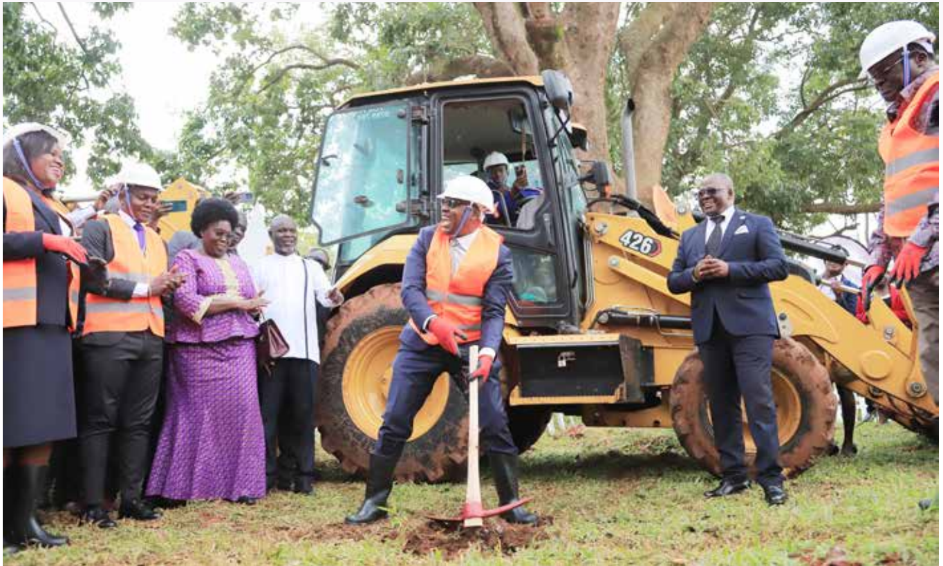
Then Deputy Chief Justice, Hon Dr Flavian Zeija, breaks ground during the groundbreaking ceremony for the Gulu Appellate Court, on July 23, 2025, as judicial officers look on.
